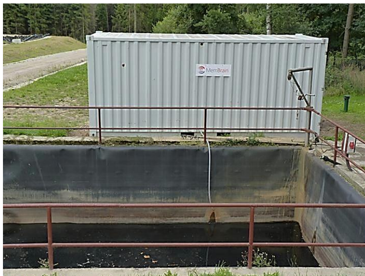
Figure 2: The container with MemBrain technology line for the landfill leachate treatment
