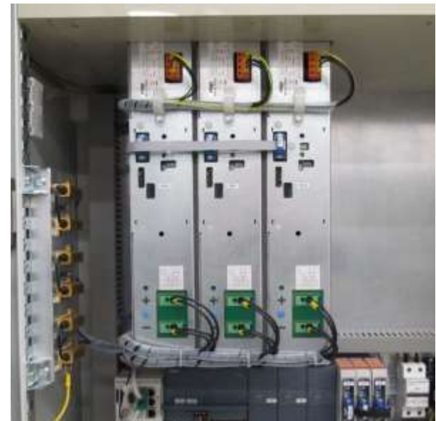
Rectifiers inside an electrical cabinet
