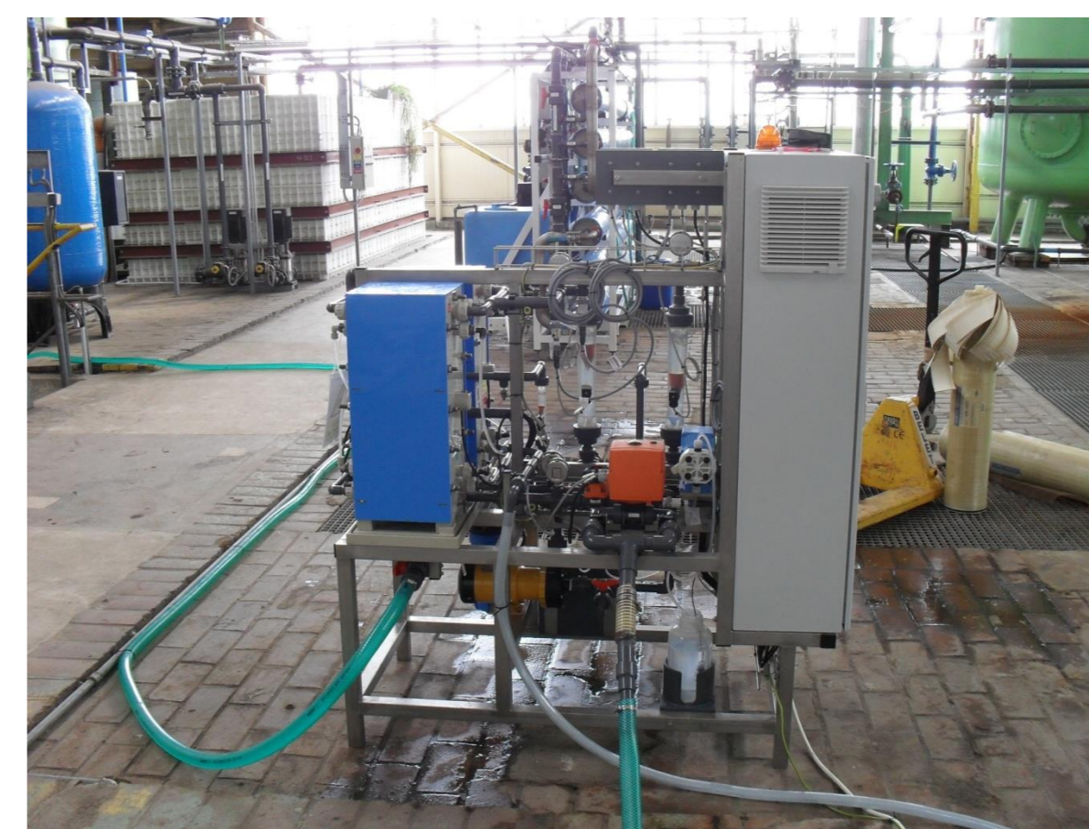
2 m 3 /h EDI pilot system at a thermal power station
